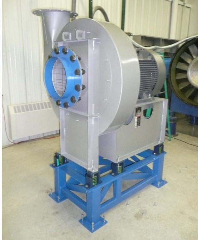
Fig. A.3 Centrifugal blower installed in the Aerodynamics Research Lab.
